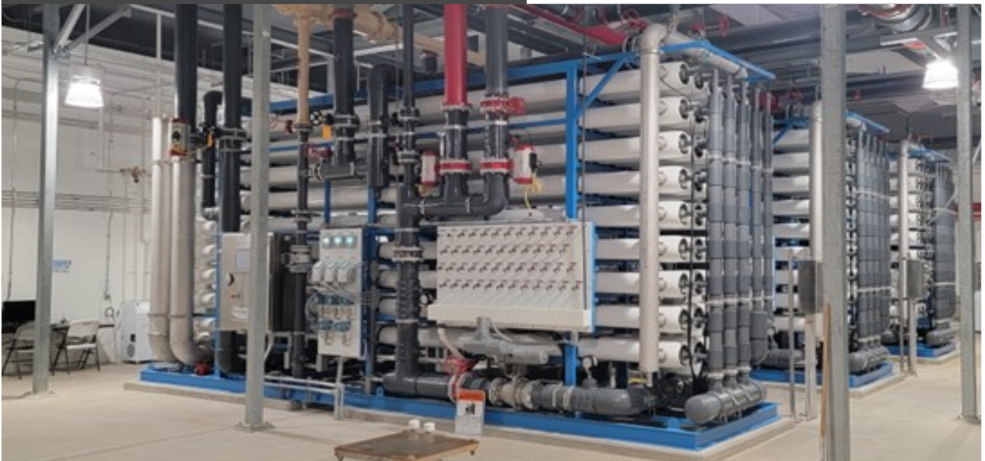
Nanofiltration treatment process at the Richard Renneker Water Plant
