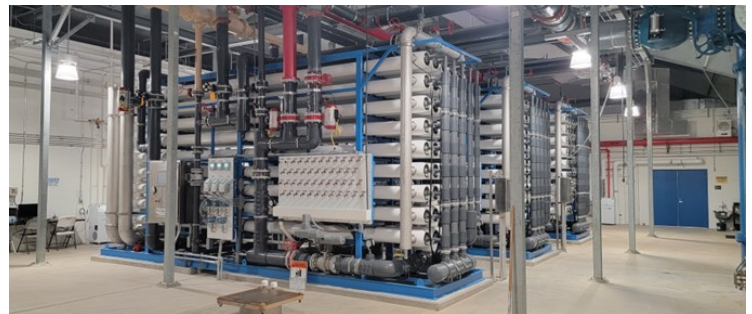
Nanofiltration treatment process at the Richard Renneker Water Plant
