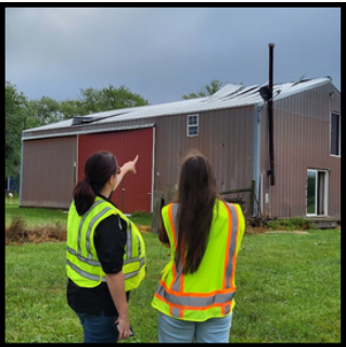
Damage Assessment with EMA's Intern on July 30th
